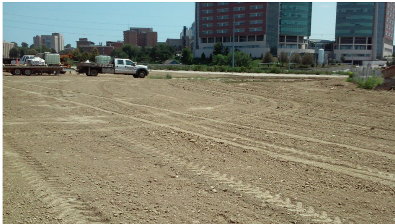
This photo shows the final grade of the former Omaha Steel Castings site following completion of remedial activities. Remedial activities included excavation of contaminated soils, removal of several underground storage tanks and building foundations, and placement of clean soil in excavated areas. The site – conveniently located across from the University of Nebraska Medical Center – is now ready to be redeveloped for new residential housing and commercial businesses.
