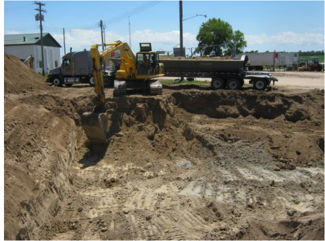
Pictured above -- Excavation of fuel-contaminated soils to allow construction of a strip mall over this area in Greeley.
