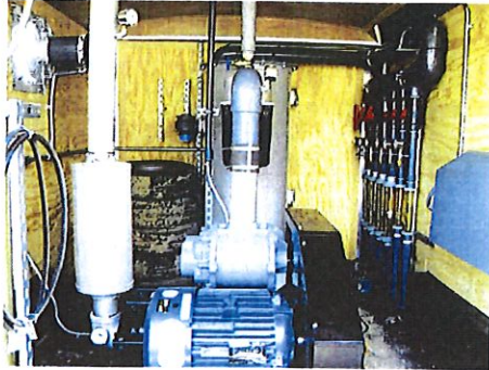
SVE blower, water knockout, Pipe manifold and tires inside The trailer.
