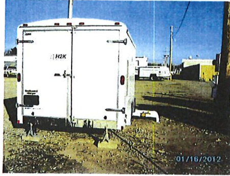
Remediation system in Trailer on site. 1/16/12
