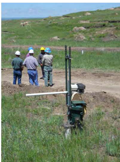
Monitoring well at CBR
