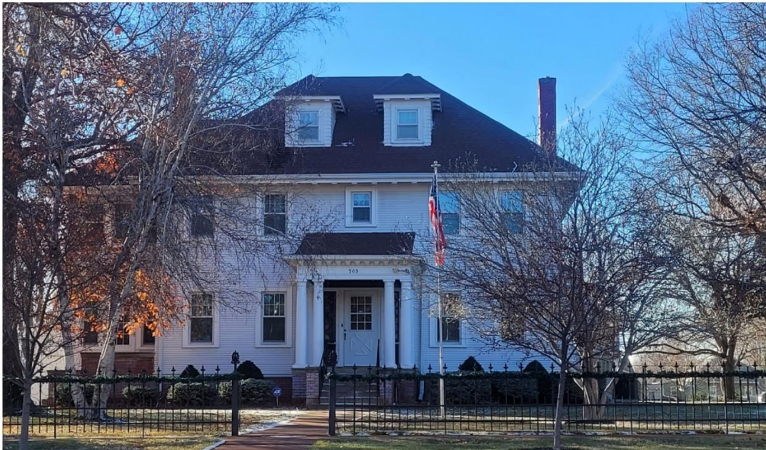
New energy efficient windows installed with funds from the Dollar and Energy Saving Loan Program (2022).
